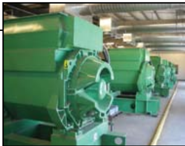
Ox Mountain LFGTE Plant. Photo(s) provided by Ameresco, Inc.
